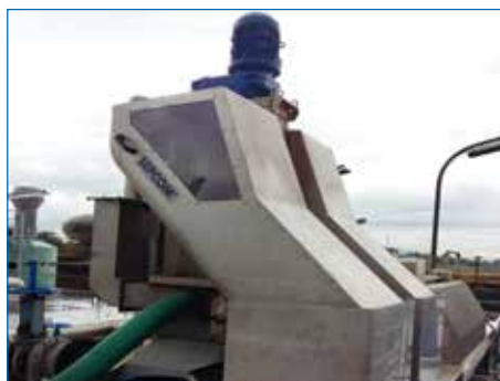
Waste water treatment plant (SEPCOM Industrial Vertical)
